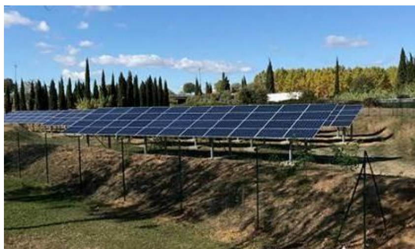
Figure 4. Illustration des panneaux photovoltaïques
