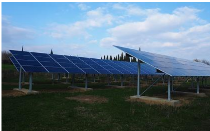
Figure 3. Illustration des panneaux photovoltaïques
